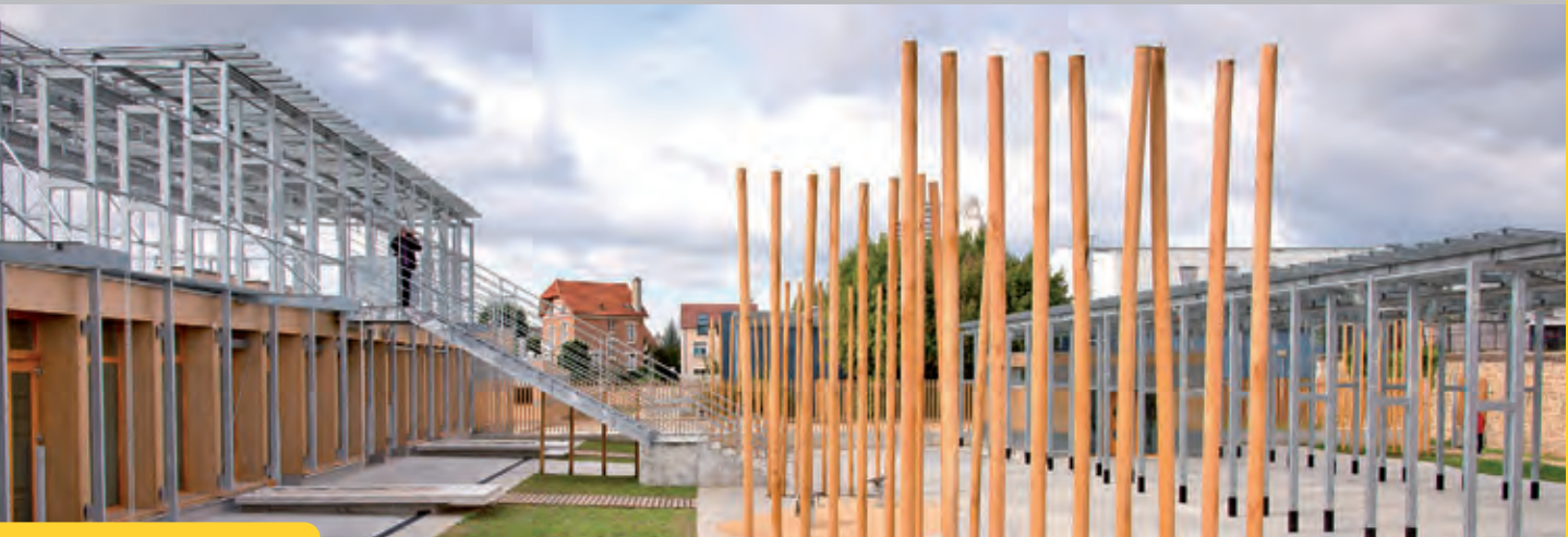
The Louise Michel School in the Fort d'Issy eco-district, first public establishment build with timber frames and insulate with straw bales. Photo credits ISSY MEDIA
