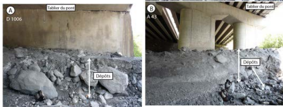
Figure 11a,b. Rieu Sec channel below the bridge of D1006 (11a) and highway from Grenoble to Turin A43 (11b).
